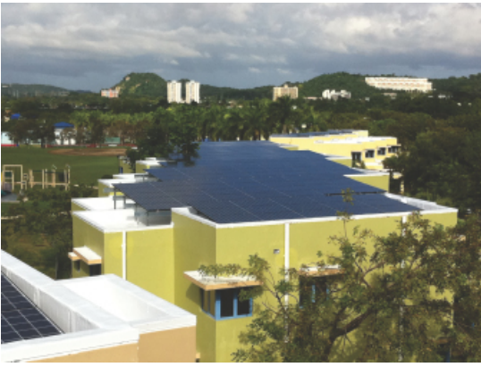
Solar Panels financed by Hannon Armstrong on roof of building at the U.S. Coast Guard Base in Puerto Rico
