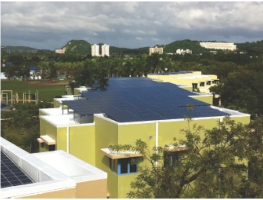
Solar Panels financed by Hannon Armstrong on roof of building at the U.S. Coast Guard Base in Puerto Rico
