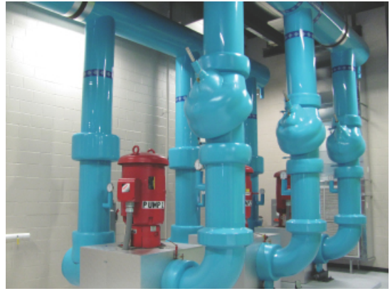
Piping at Chiller Plant financed by Hannon Armstrong for a large urban hospital
