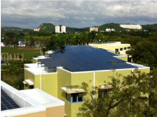
Solar Panels financed by Hannon Armstrong on roof of building at the U.S. Coast Guard Base in Puerto Rico
