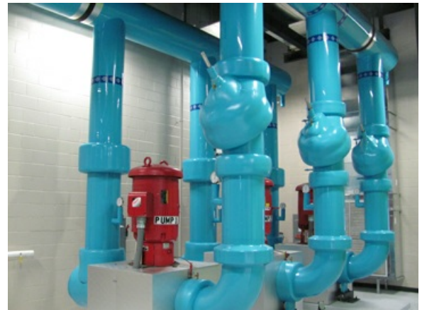
Piping at Chiller Plant financed by Hannon Armstrong for a large urban hospital
